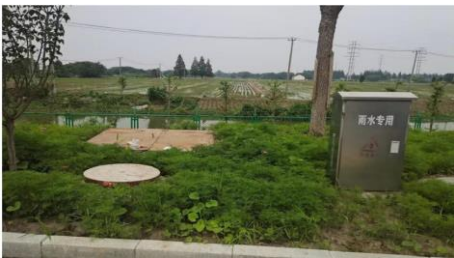
Rainfall Collection System at Luxshare Electronic Kunshan
